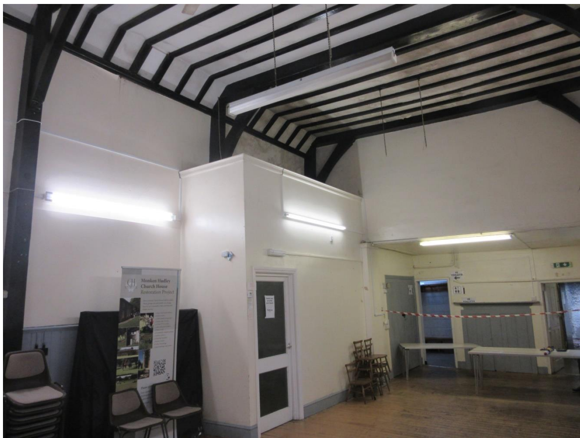
Figure 24: The interior looking north, with modern stair enclosure and doorways to north extensions.
